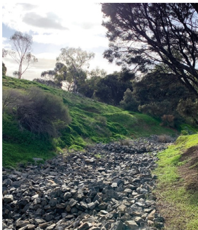
Figure 7. Excessive watercourse rock lining.
