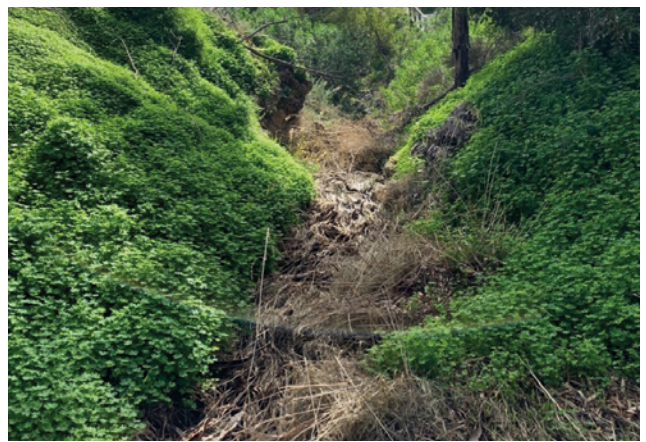
Figure 13. Erosion in Barton Gully.
