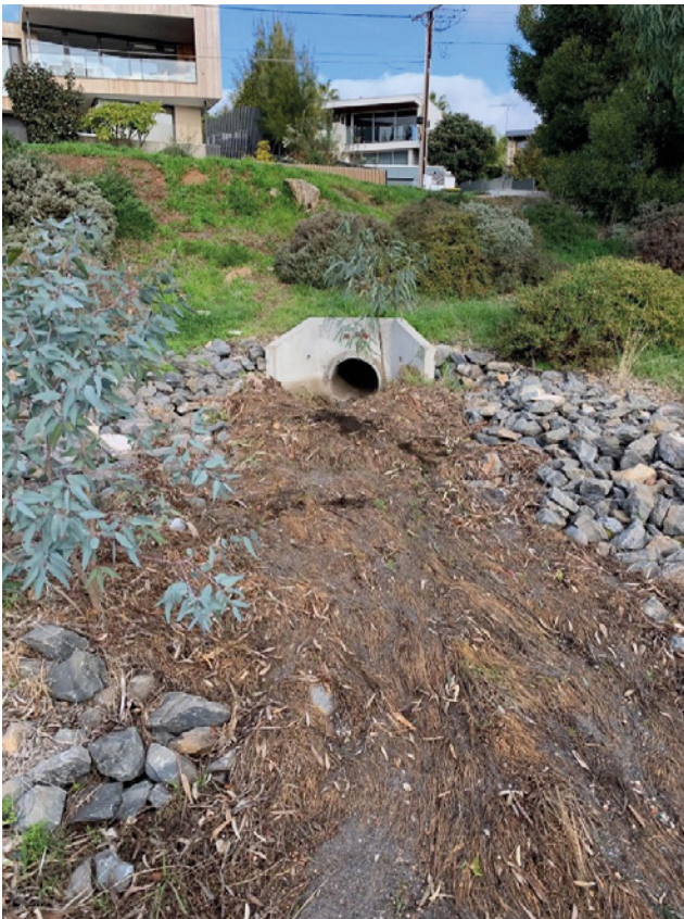
Figure 12. Barton Road stormwater discharge into Barton Gully.
