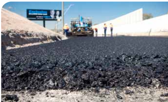
Warm Mix Asphalt is produced and laid at a temperature range from 110 - 140°C, much lower than traditional asphalt products.
