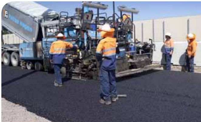
Warm Mix Asphalt has been used to great benefit by Fulton Hogan as part of Origin Alliance's upgrade of the Ipswich Motorway project in south east Queensland.
