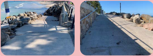
Site 6 - High due to potential safety issues
