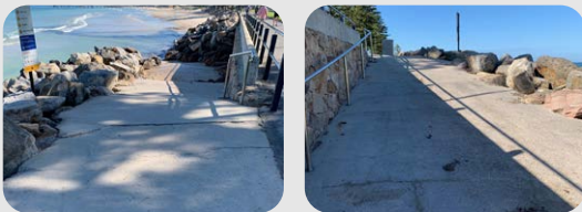
Site 6 - Large non-compliant ramp
