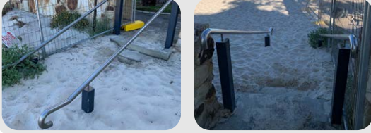
Site 1 - Redundant stairway buried in sand
