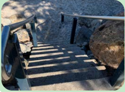
Site 5 - Low due to trip hazard not being too significant
