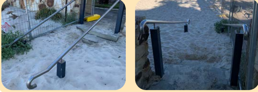
Site 1 - Medium due to trip hazard
