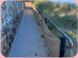
Site 4 - High due to persistent maintenance requirements
