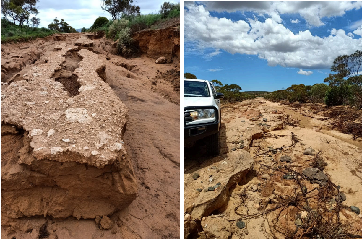
Figure 1: Examples of damages to roads following ex Tropical Cyclone Tiffany.
