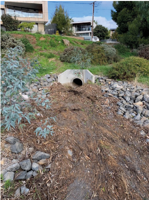
Figure 12. Barton Road stormwater discharge into Barton Gully.
