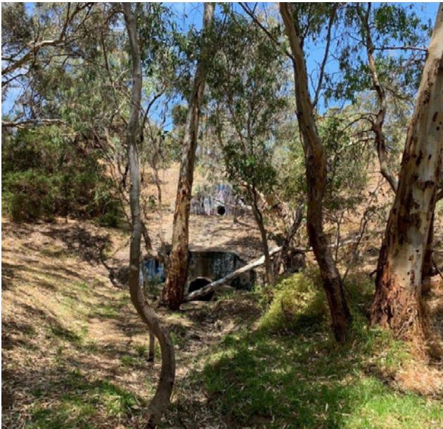
Figure 11. Upstream drainage infrastructure.
