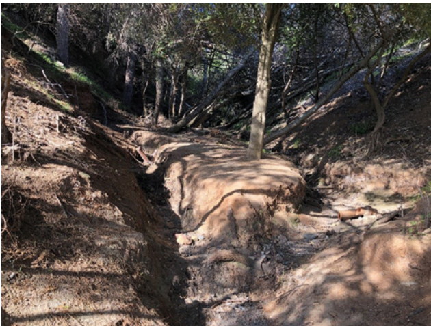
Figure 3. Erosion on steep embankment.
