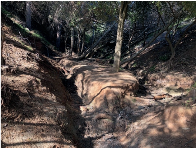
Figure 3. Erosion on steep embankment.
