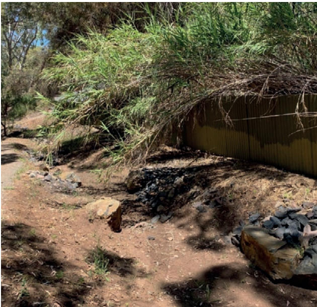
Figure 14. Erosion along drainage line.
