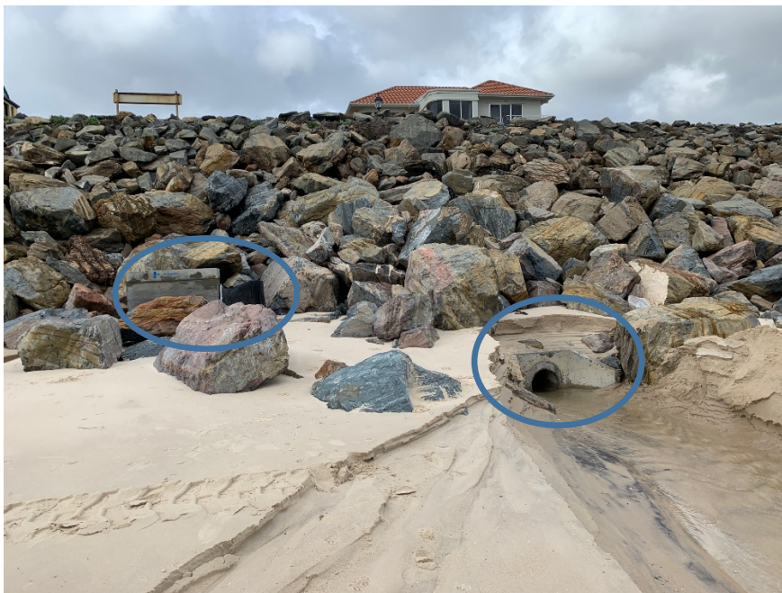
Photo 1- Bickford Terrace outlet below normal sand level with high level outlet to left
