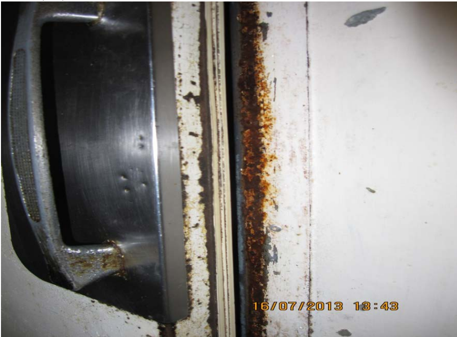
Figure 8: Rust and worn paint on the cold room floor door — effective cleaning not possible.
