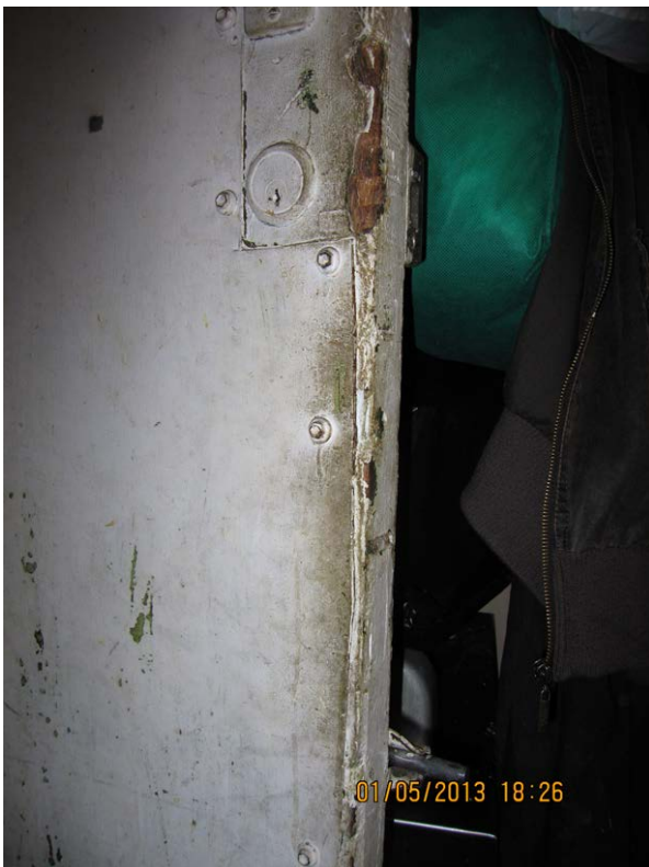
Figure 4: Back door, the hand contact surface of the door is dirty and conducive to cross-contamination of food. The surface of the door is not able to be effectively cleaned.
