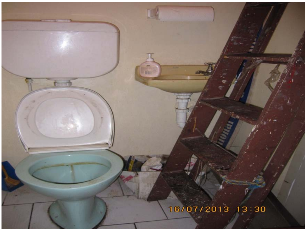
Figure 7: Non-complying hand basin (no supply of warm water). Access to the hand basing blocked.
