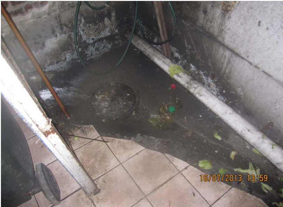
Figure 10: Floor drain (contained within a closet in which the rubbish bins are stored).
