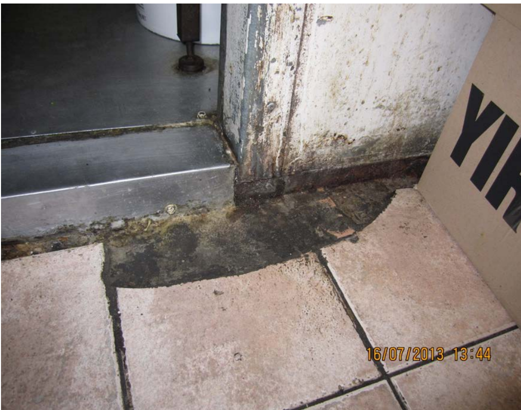
Figure 9: Damaged floor; dirty areas of the floor & cold room.
