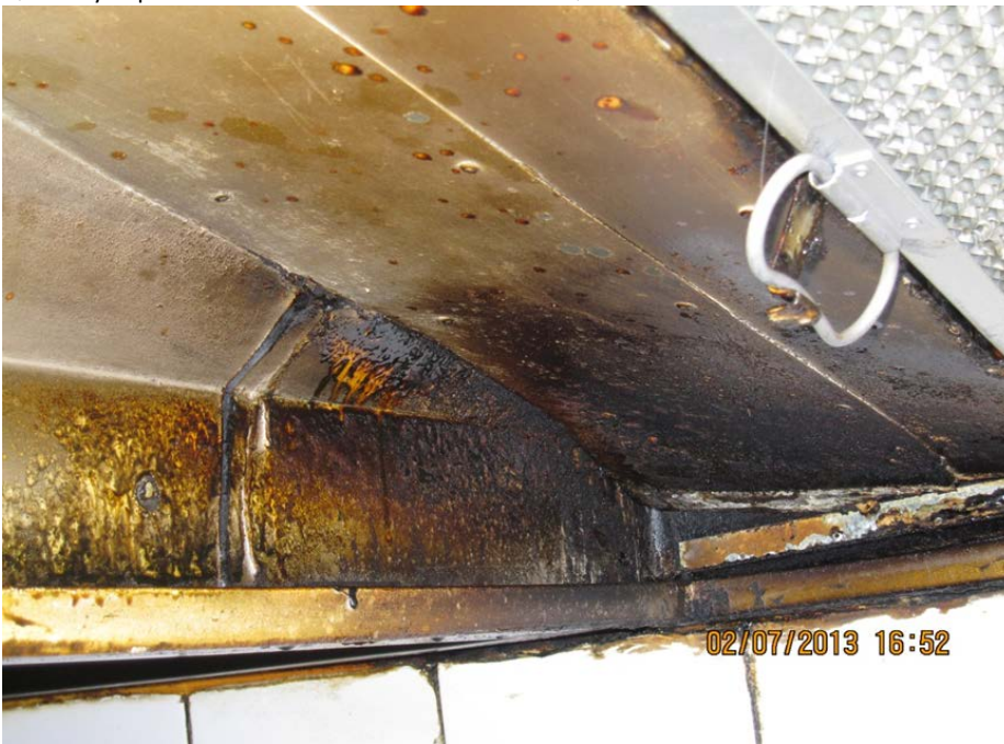
Figure 5: Section of the exhaust canopy on which grease has built up.
