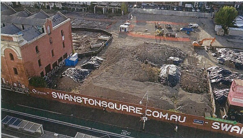
The site of last Thursday's wall collapse, pictured in 2012, has seen a procession of failed developments since being cleared. Photo: Glenn Wilson
