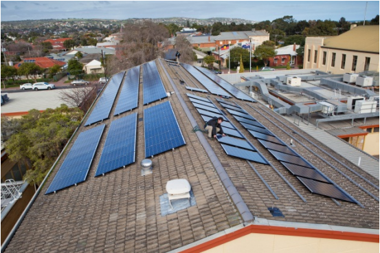
Figure 1 – 46 kW solar power at the Civic Centre
