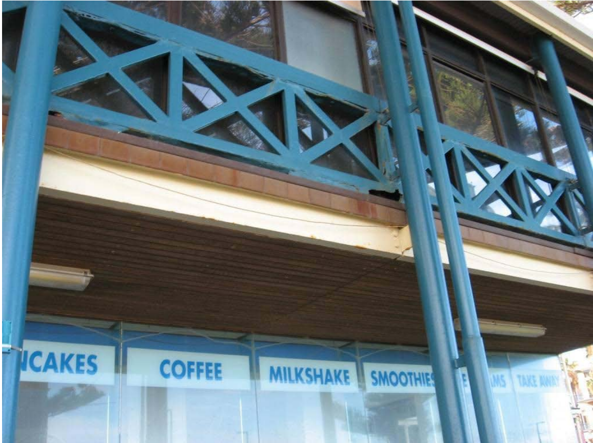
Photo 1 – External Balcony – corrosion to Support Steelwork and Balustrade
