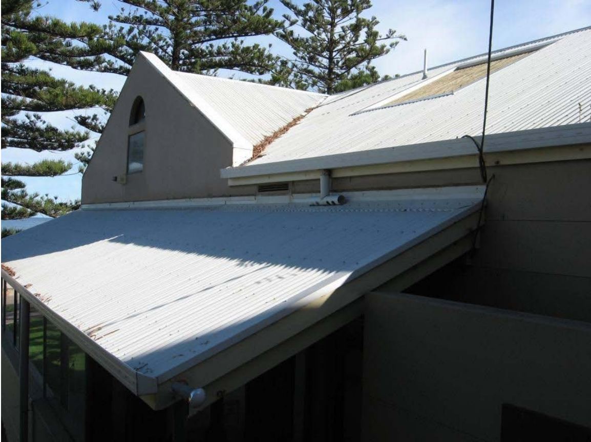
Photo 2 – Debris on southern side of roof
