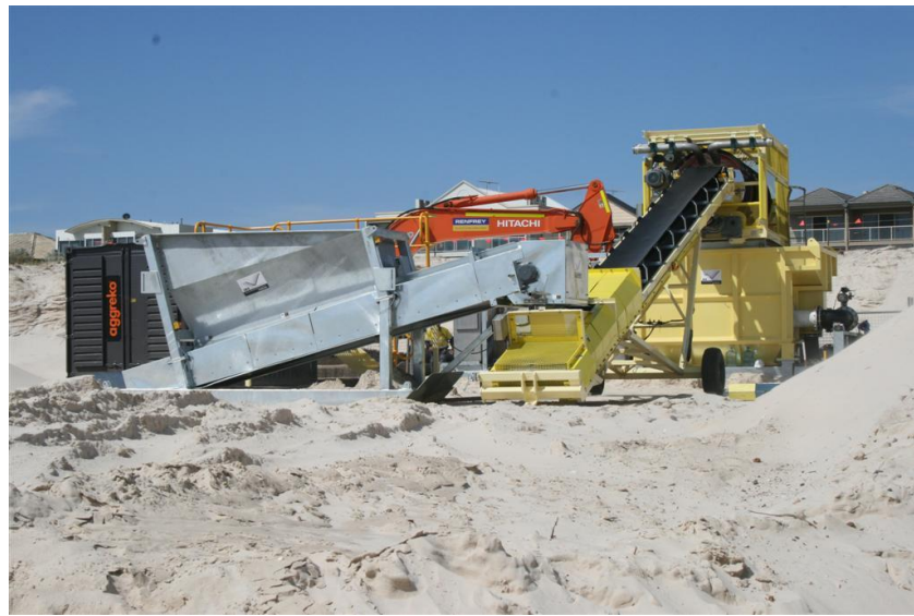
Sand Collection Unit commissioning at Torrens Outlet in November 2012.
